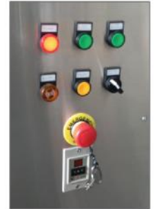
Local digital panel control
