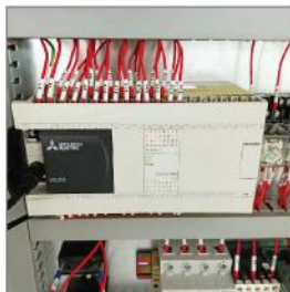
Mitsubishi local PLC brand
